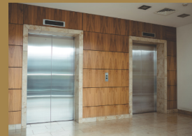
Schindler or Equivalent Brand Lift with 24 Hours Power Backup
